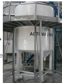
Satellite Hydration, (close to customer)
