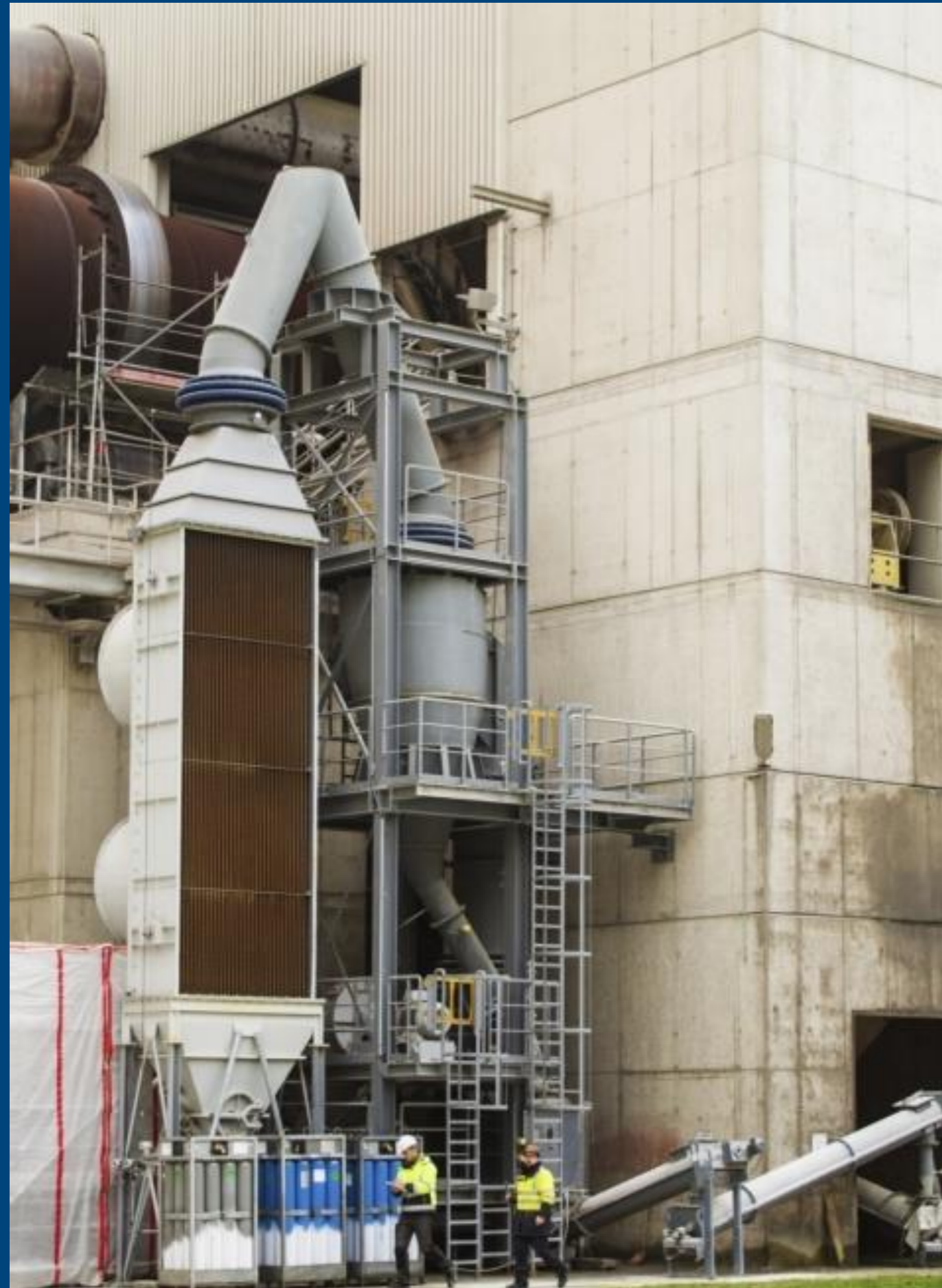
Fig.1) Oxyfuel clinker cooler prototype (TRL6) tested in the HC cement plant in Hanover.
