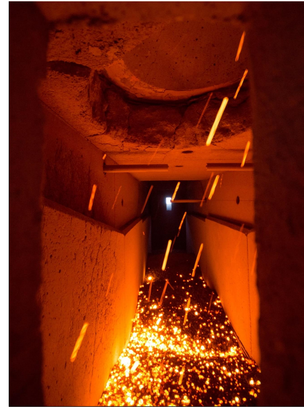
Fig.4) Inside view of the oxyfuel clinker cooler prototype during the trials
