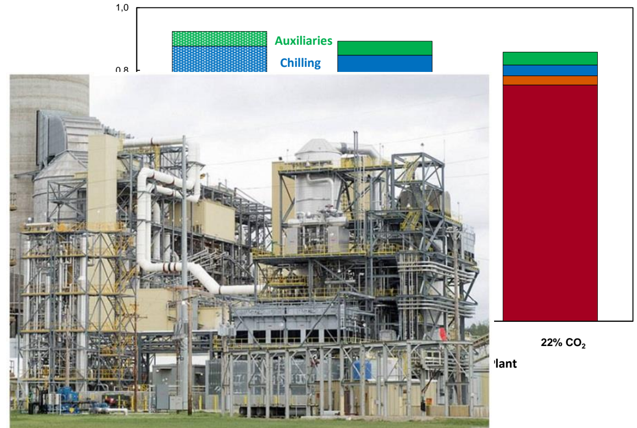
Product Validation Facility at the Mountaineer power plant, WV (50 MW th ):8000 h in 2009-2011
