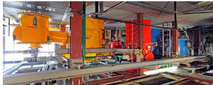
Alstom Power Calcium Looping – TRL 3
