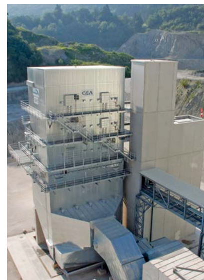
Figure 1: SCR facility in a cement works
