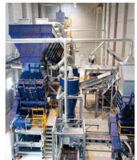
Figure 2: Example of a modern pre-treatment facility
