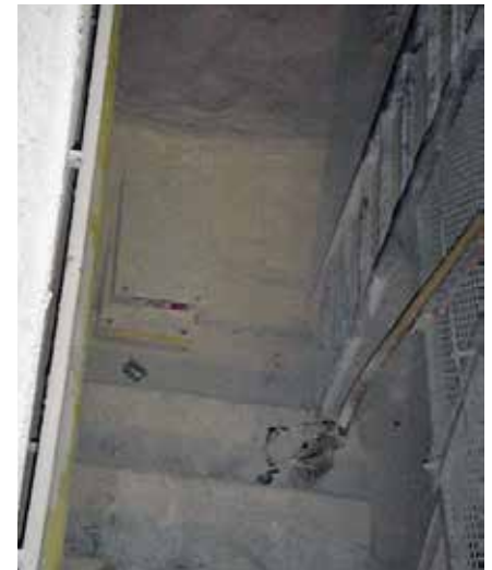
Figure 2: Basement area after an escape of hot meal.
