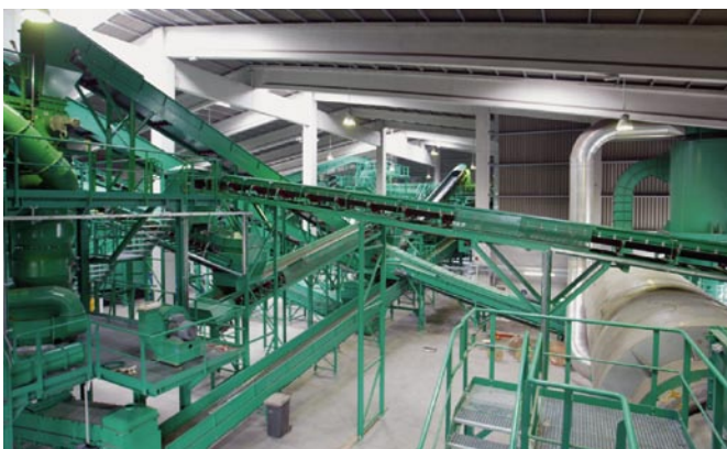
Fig. 1: Modern plant for the pretreatment of waste fuels (Source: Ecowest)
