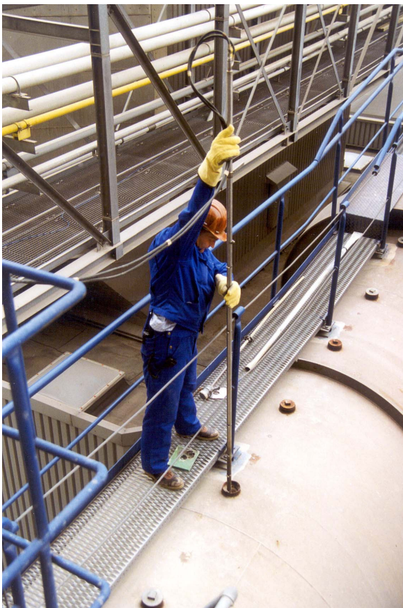
Fig. 1: Measurement of tertiary air volume flow
