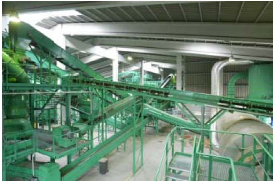
Fig. 1: The pretreatment of mixed waste fractions to get a suitable fuel requires various processing steps.
