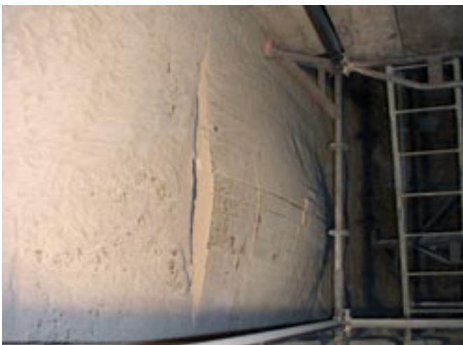
Fig. 1: Lining detached due to insufficient clearance between expansion joints
