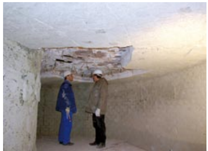
Fig. 2: Cyclone ceiling segment fallen out
